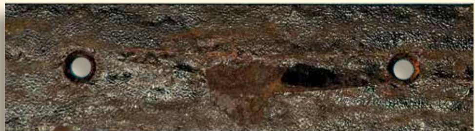
Close up of Deliberate Scratch shows excessive rust, dramatic rust migration, and advanced detachment of the surface coating
